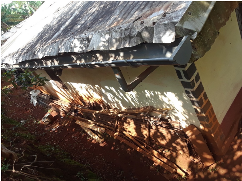
Figure 19 - Rainwater catchment system, roof and gutter view. Photo taken on my phone, June 2018. Point labeled "WaLi Water Collection System" on map
