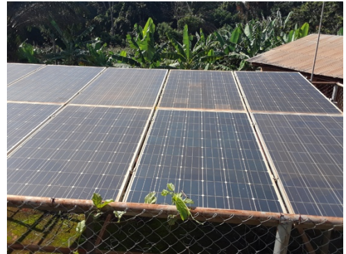
Figure 25 - Solar panels of the solar power water system in Batoufam.
