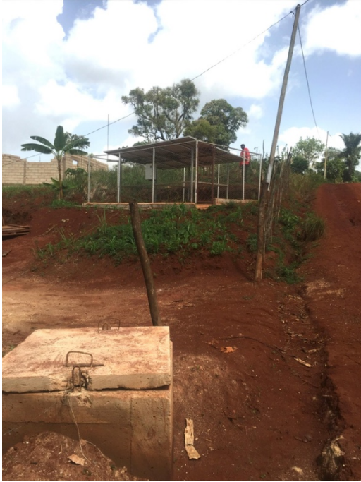
Figure 26 - Solar powered water system, photo of well (concrete box) and associated solar panels. Source: photo from my phone
